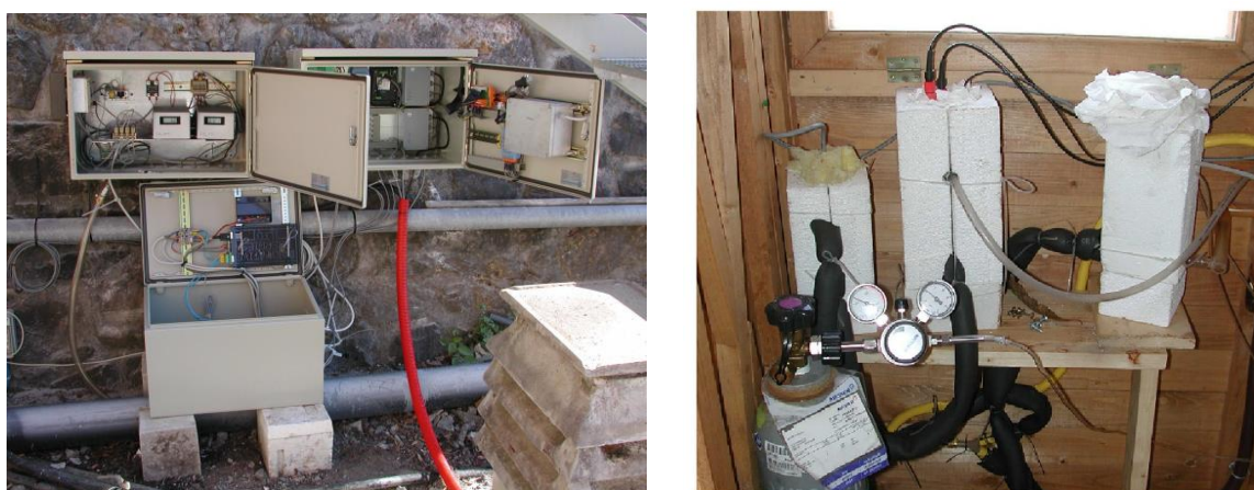
Fig. 2. The IGG-CNR-Pisa continuous automatic monitoring stations: left) cupboards containing the electronics. right) Cells dedicated to physicochemical water parameters and to the concentration of dissolved gases measure.
